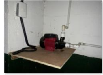
New water pump
